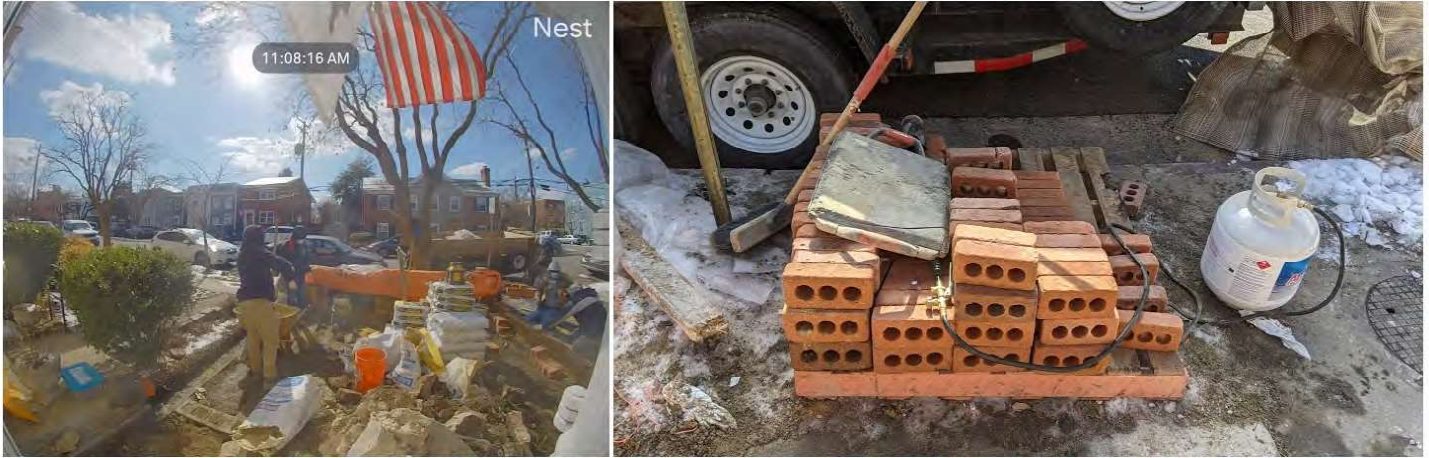
Day 5 Feb 20: Brick walls are being installed. Due to below freezing temperatures, a torch is being used to heat the bricks and grout for installation.
