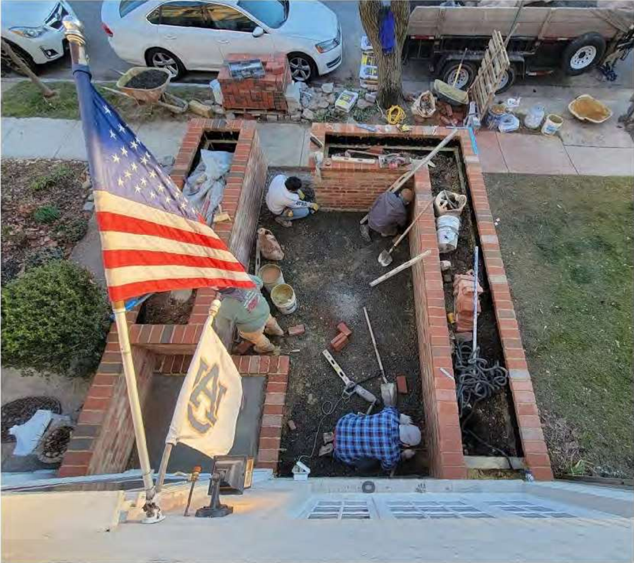
Day 8 Feb 25: The crew installed the brick topper and began pad prepping. Then, we worked on finishing installing the lights.
