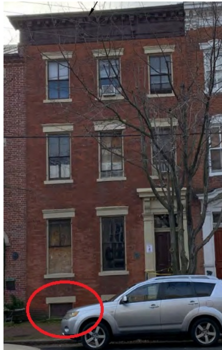
Figure 2: Front elevation with cellar window circled. Other cellar window obscured by car.
