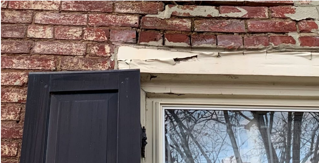
Figure 2: Type of damage that can be associated with water damage to historic brick
