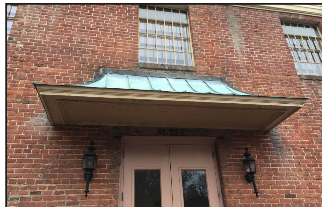
Existing Entry Canopy to be Removed
