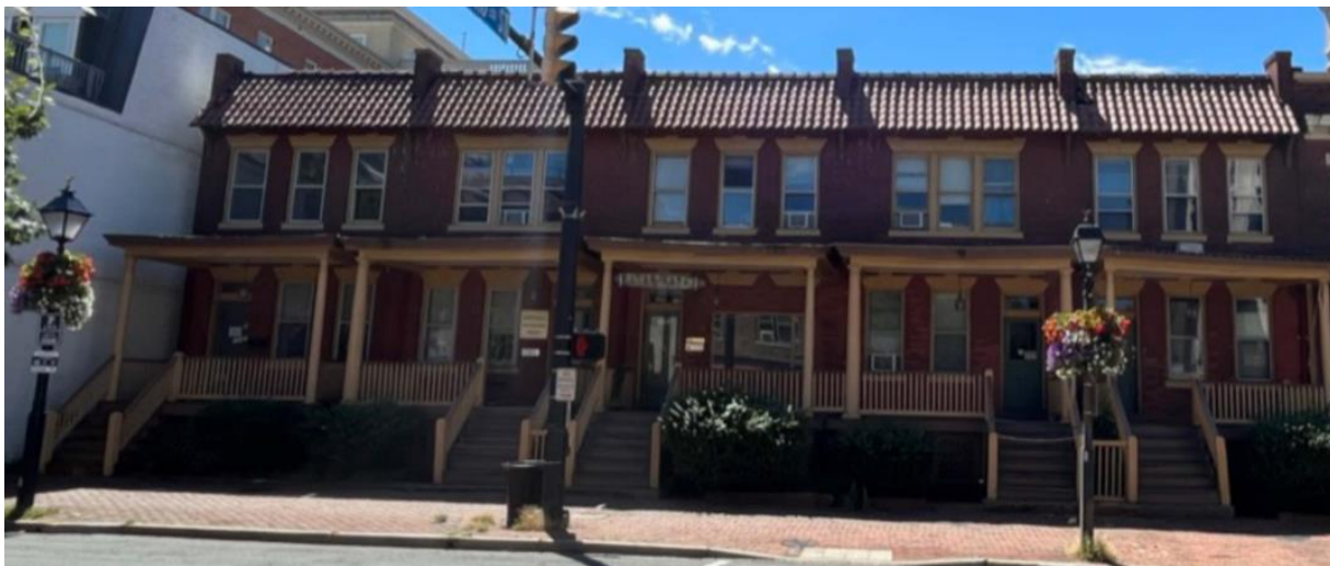
Figure 7: North elevation of 1604-1612 King Street, noting the tile roof and expressed party walls
