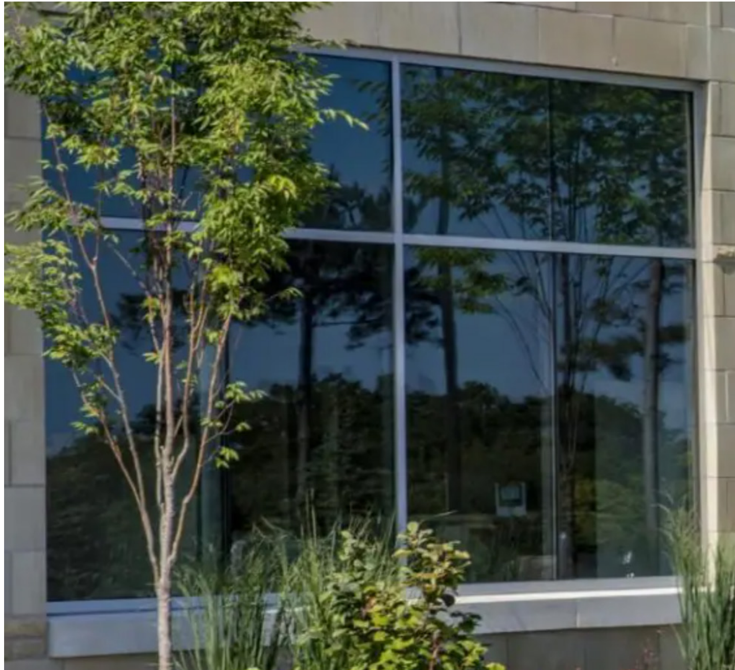
NEW WINDOWS AND FRAME TO MATCH MULLION FACE WIDTH, GLASS TYPE AND SILICON VERTICAL JOINT
