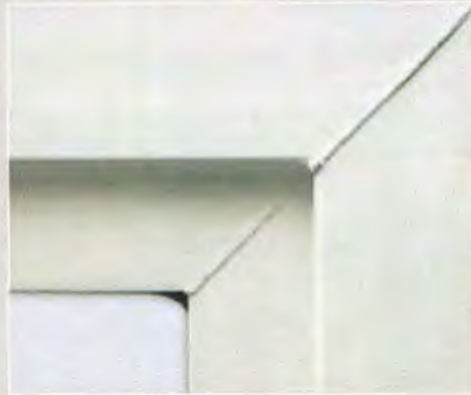
Typical welded vinyl corner seam with distracting ridges
