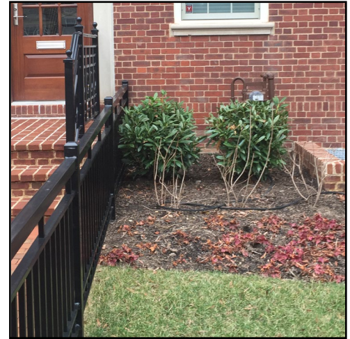
Meter may be located on the façade behind a landscape screen. Paint meter to match the adjacent wall color.
