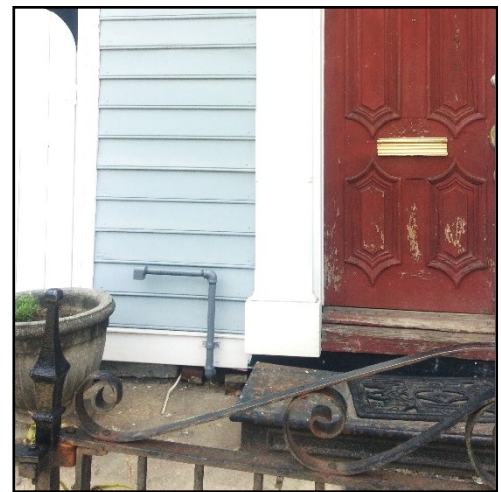
For existing structures, meter may be placed on front façade if it is a safety risk to be located elsewhere. A pressure relief vent may be located on the front or side façade. Paint all to match adjacent wall color.
