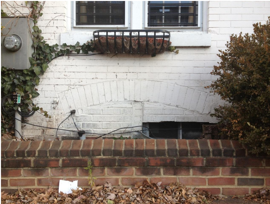
Figure 1: Photograph of 1109 Duke Street basement window. Identical to 1107 Duke Street, except that the basement opening at 1107 Duke Street is completely bricked-in.
