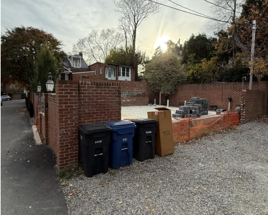
View from rear NE corner of property (proposed garage location) looking down to Duke Street.
