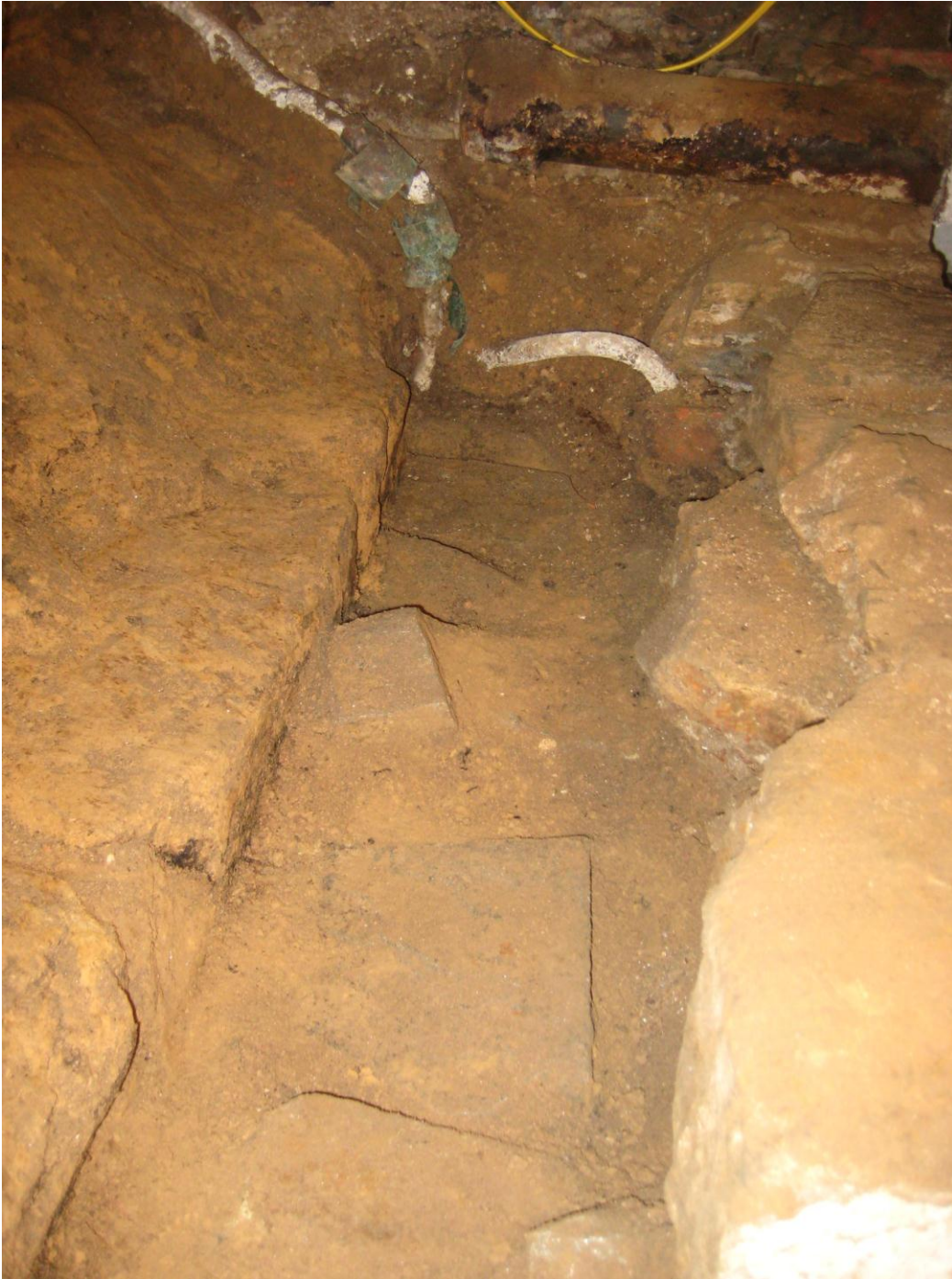
Figure 7. Detail showing the relationship of the natural clay subsoil, the builder's trench comprised of mixed sandy clay and stone, and the top of the north cellar wall after the top courses were removed. The iron drain pipe and a defunct lead water line are visible in the background.
