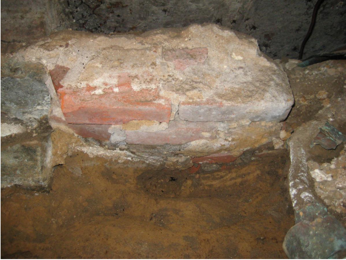
Figure 6. Detail of the two-brick-wide arch, bonded into the stone fireplace base. The area to the right of the arch has been disturbed by later construction.
