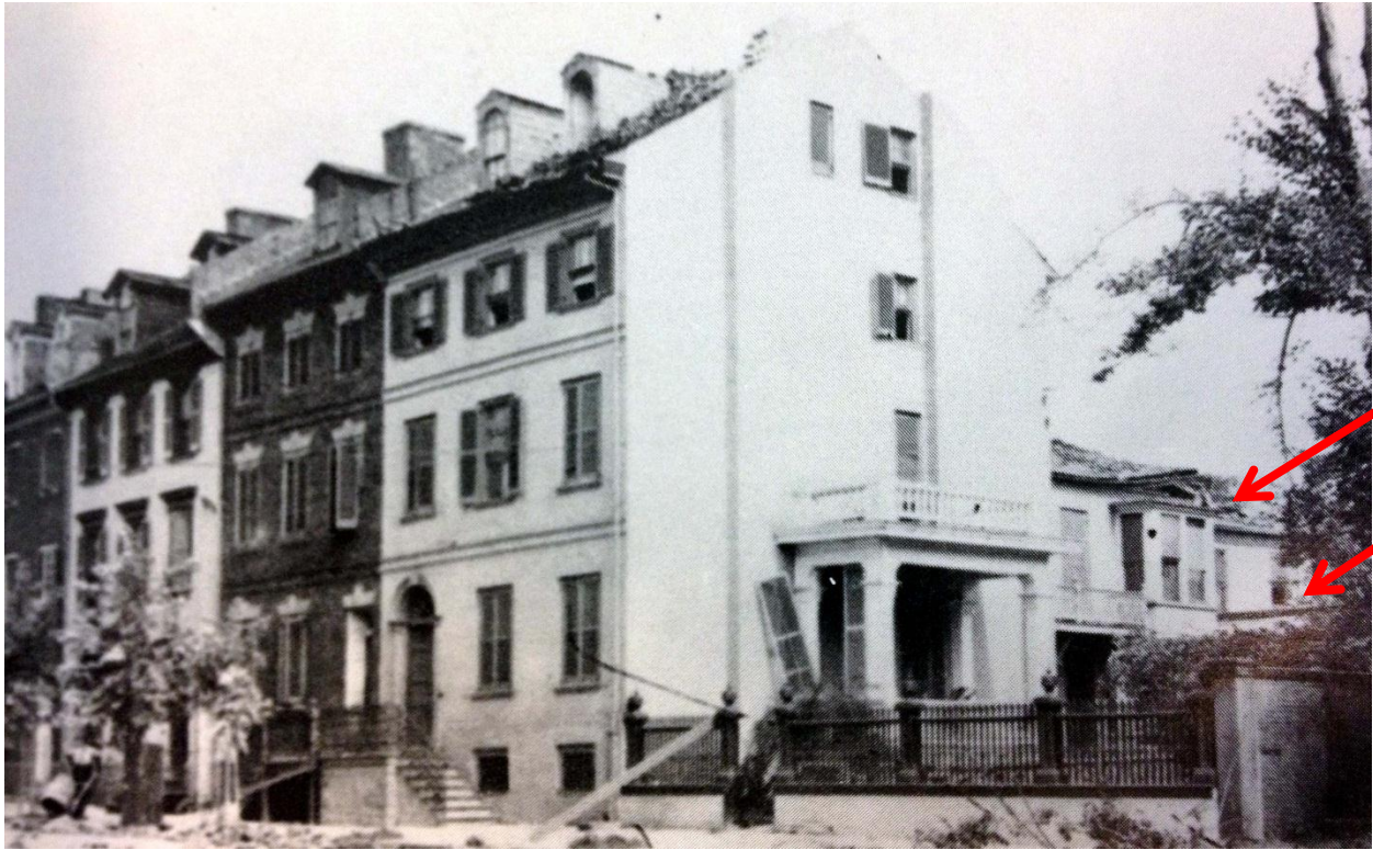
Figure 3: 207 Prince Street, circa 1913 showing damage from a severe windstorm. Note the additions on the east elevation. Image taken from A Seaport Saga: Portrait of Old Alexandria, Virginia by William Francis Smith and T. Michael Miller
