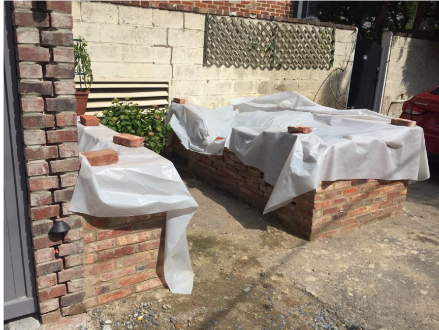
Figure 3 Current condition of the proposed planters. No additional work has occurred on the site since the stop work request was issued.
