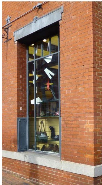
Figure 5. 326 King Street (upper left), 206 South Union Street (upper right), and 201 King Street (above) for modern storefront windows. 201 King Street has a granite sill, significant jamb depth and traditional details including the cast iron lintel, jamb guards and star washers.
