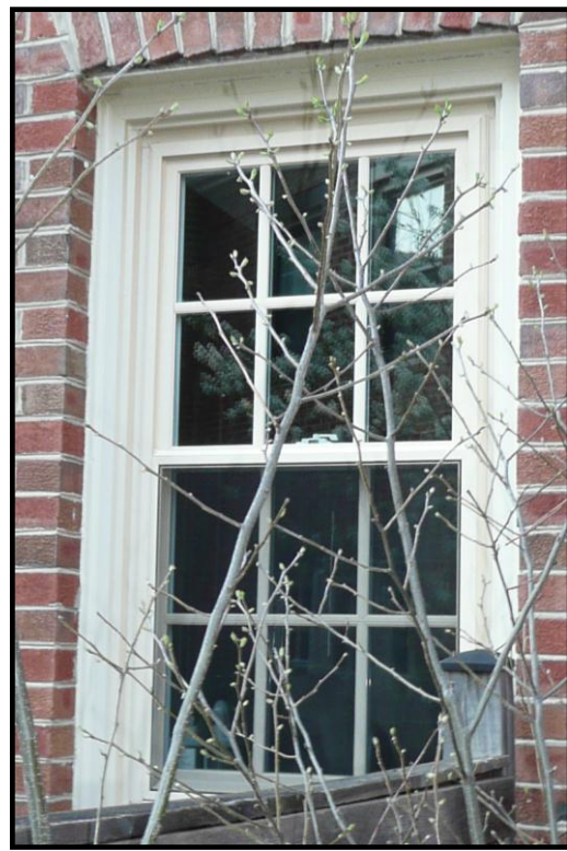
Figure 2: Photo of Installed Vinyl Insert Windows
