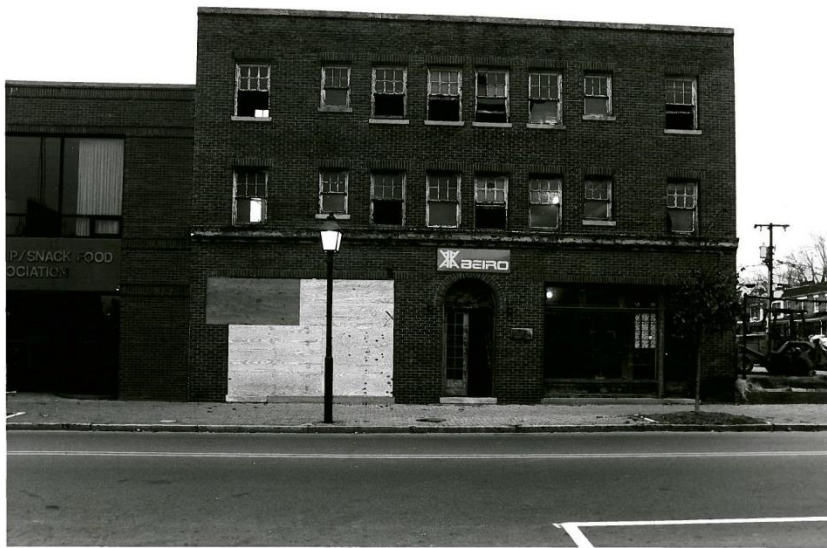
NAVAL RESERVE ASSOCIATION HEADQUARTERS RENOVATIONS ALEXANDRIA, VIRGINIA A. A. BEIRO CONSTRUCTION COMPANY GENERAL VIEW LOOKING NORTH DECEMBER 14, 1984
