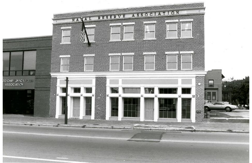
NAVAL RESERVE ASSOCIATION HEADQUARTERS RENOVATIONS ALEXANDRIA, VIRGINIA A. A. BEIRO CONSTRUCTION COMPANY GENERAL VIEW LOOKING NORTH JULY 29, 1985
