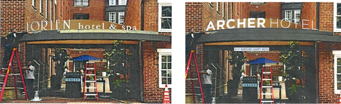
Figure 1: Existing (left) and proposed (right) canopy sign at the courtyard entrance, facing King Street
