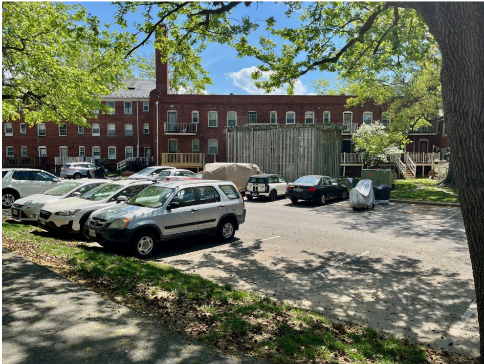
Figure 2: Existing cooling tower
