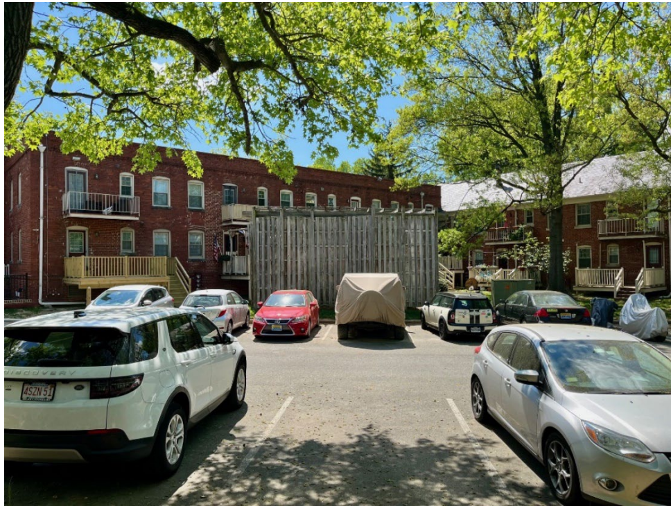
Figure 3: Existing cooling tower
