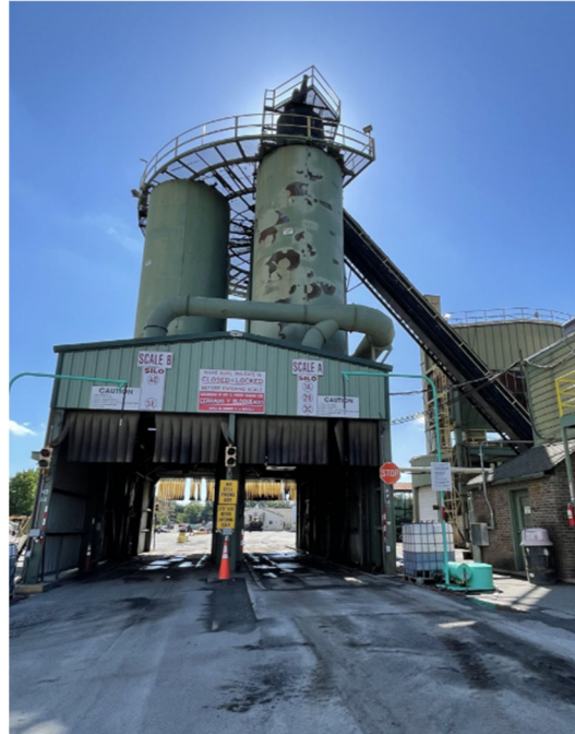
Figure 7: Asphalt loading facility
