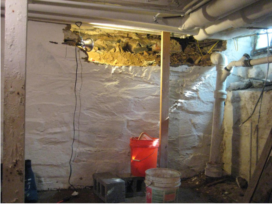
Figure 3. The east portion of the north wall after the top courses of stone were removed to allow access into the crawl space. Note the drain pipe that enters the building at the northeast corner of the north foundation and passes through the cellar.
