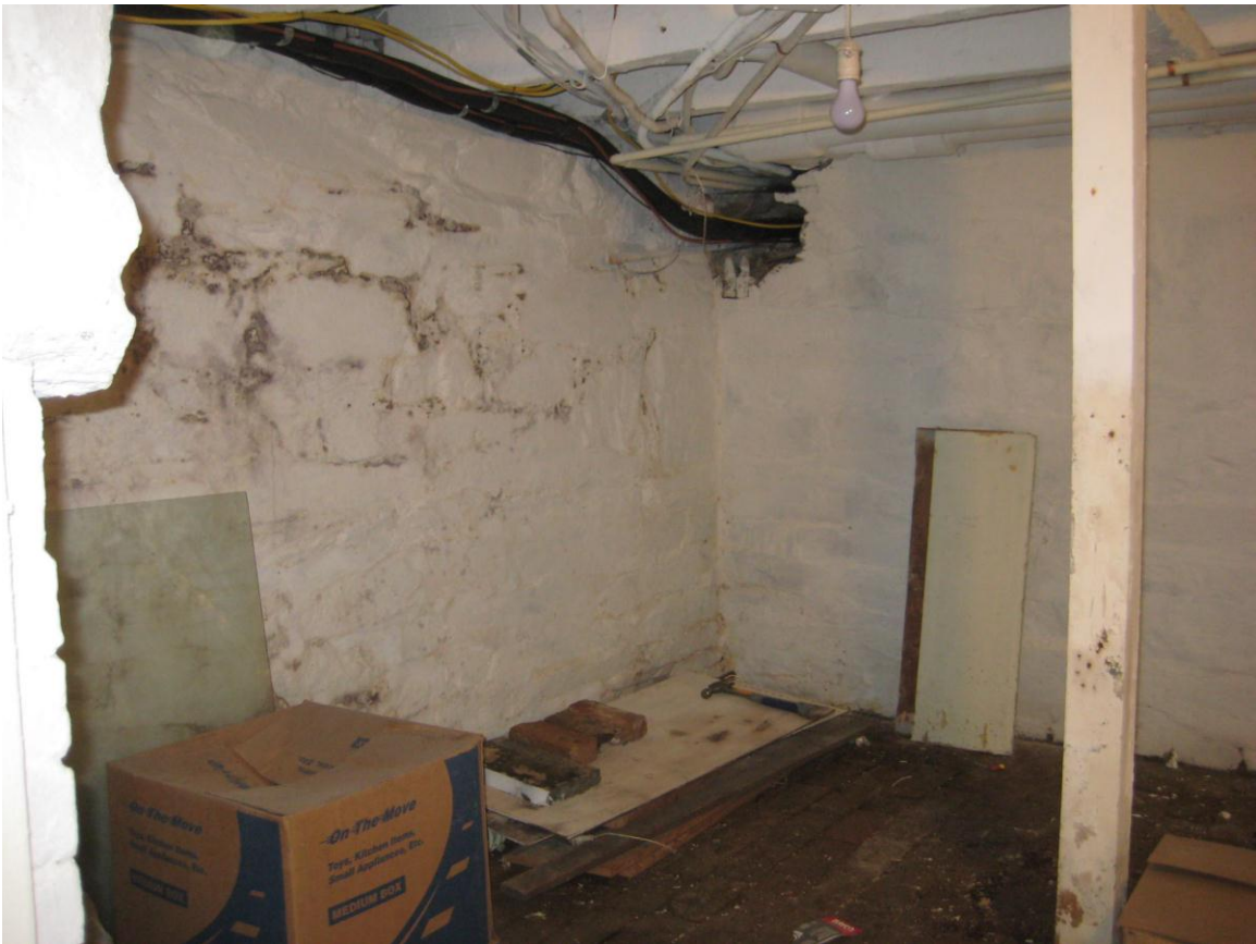
Figure 1. The kitchen cellar, showing the west foundation and the west portion of the north wall. Note the hole in the wall that has been created to accommodate various utility lines, and the relatively smooth character of the wall surfaces.
