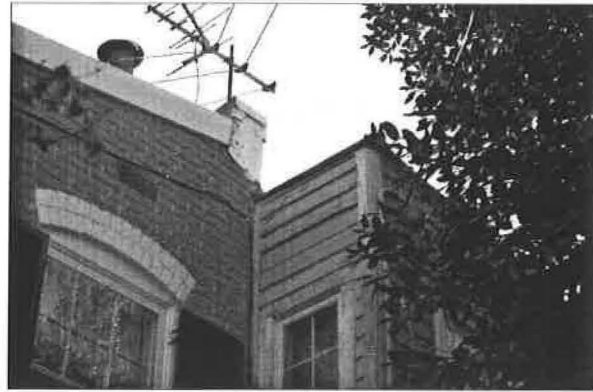
Ell of 203 S. Lee Street abutting 201 S. Lee St. ell at south property line.
