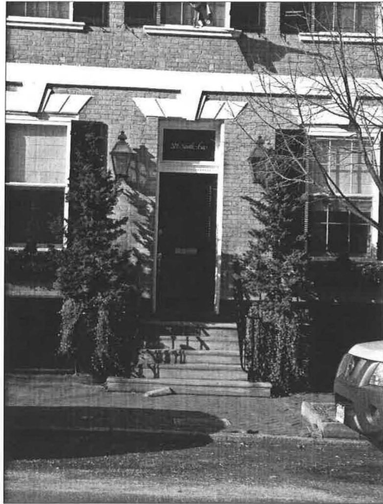
Front door facing S. Lee Street. Note brick jambs altered for a lessened-width opening.
