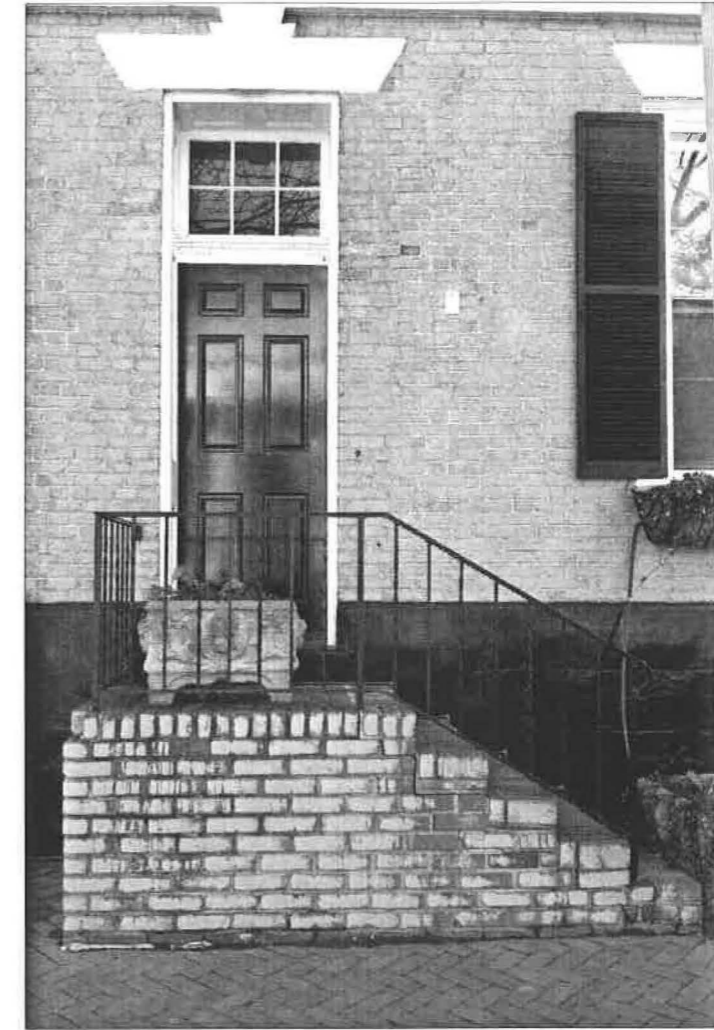
Abandoned door and stoop on Prince Street. Note brick jambs altered for a lessened-width opening.
