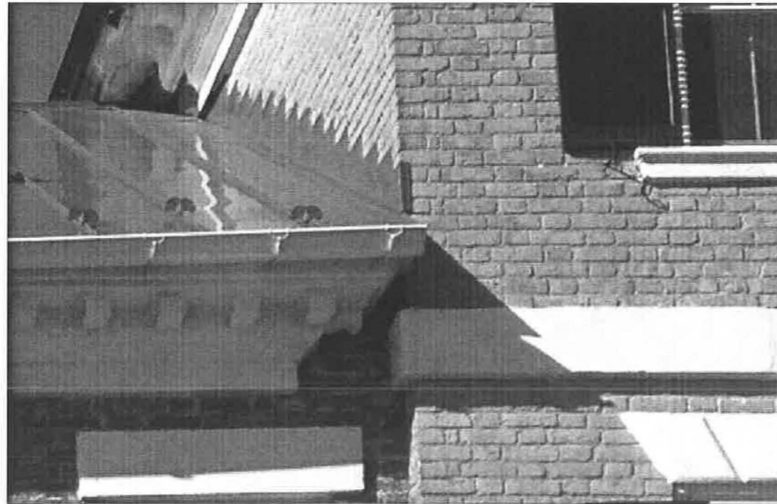
Detail of south wing cornice and roof abutting the south wall of 201 S. Lee Street.
