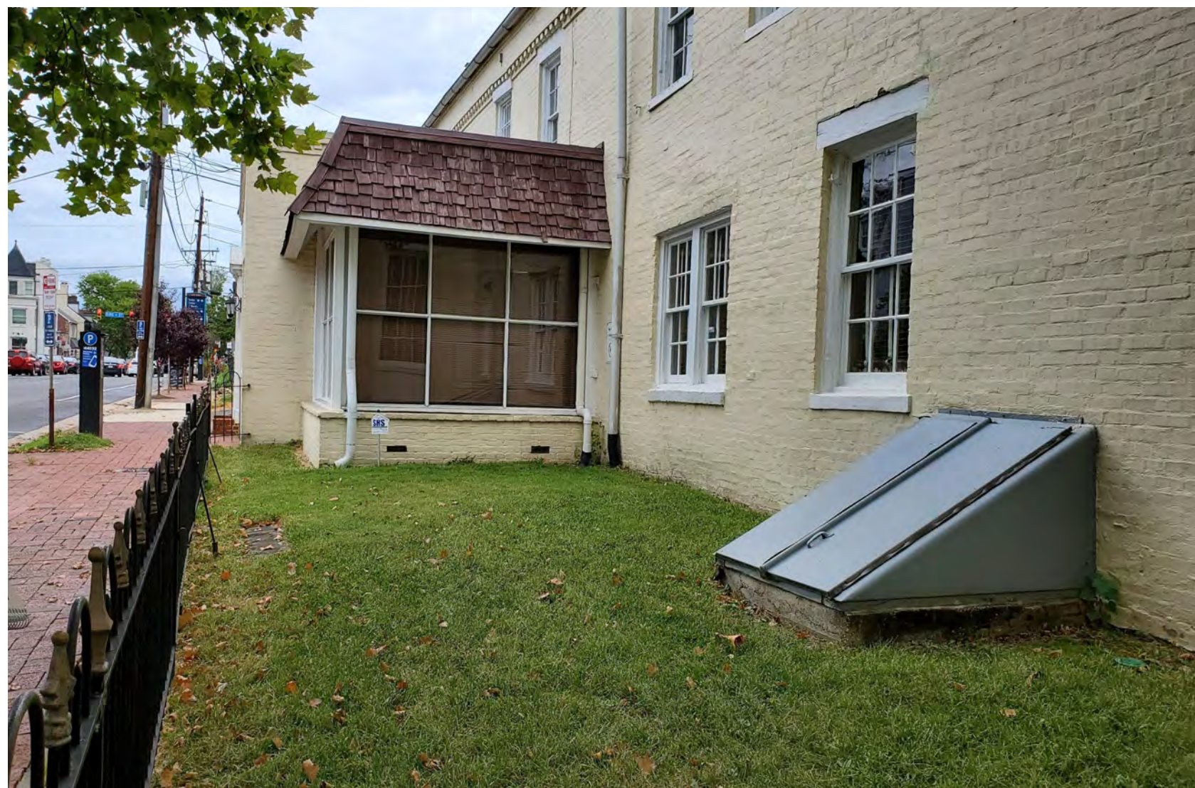
A new opening will be created at the Patrick Street enclosure. The existing iron railing will be placed on a 6" masonry retaining wall. The retaining wall will allow for regrading between the ends of north and south side yard.
