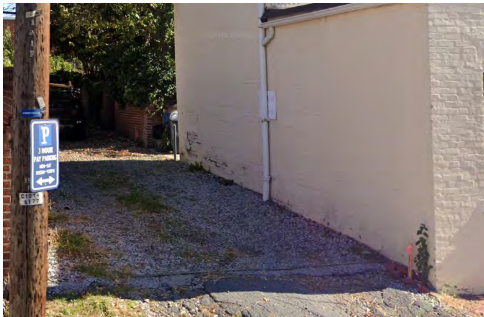
The Alley entrance driveway condition will be repaired by replacing the asphalt and crushed stone with stamped concrete.
