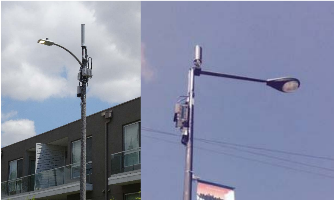
Figures 1, 2: Typical Small Cell Facility installations
