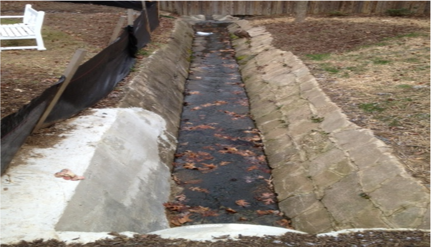
CULVERT AT 1420 KEY DRIVE...BACK YARD
