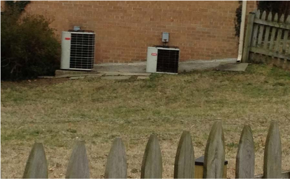
HVAC UNITS @ REAR NEIGHBOR
