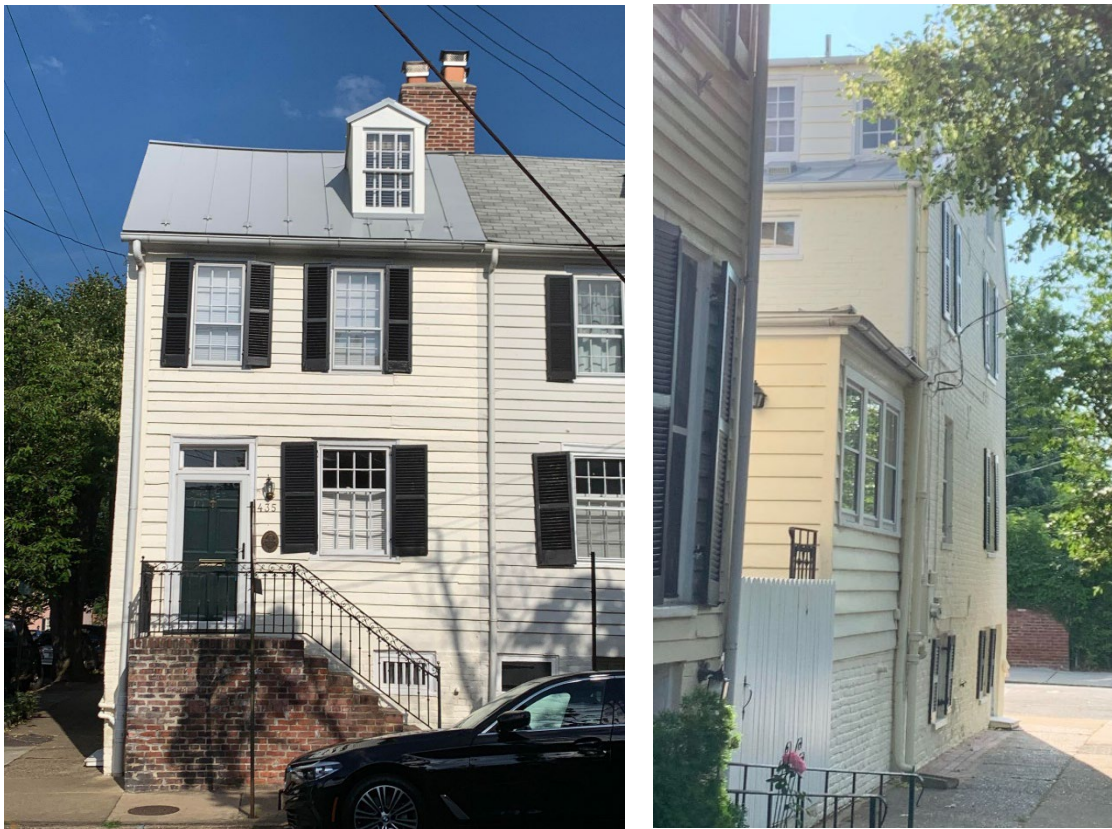
Figure 1. 435 South Lee Street with new standing seam metal roof, east elevation (left) and west elevation (right).
