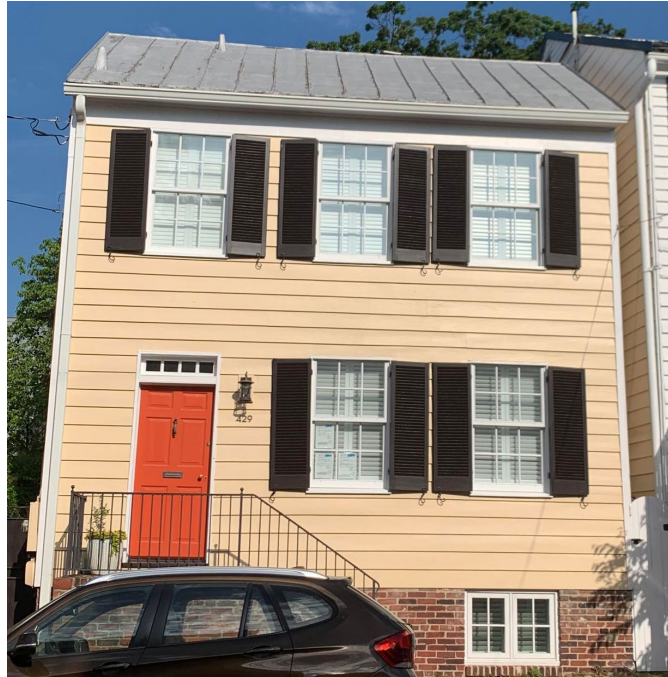
Figure 2. 429 South Lee Street, one example of an 18 th Century building on the block that now has a standing seam metal roof.
