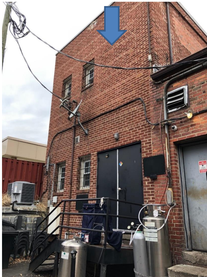
Figure 2: South/rear elevation of 610 Montgomery. Note evidence of former opening below arrow.
