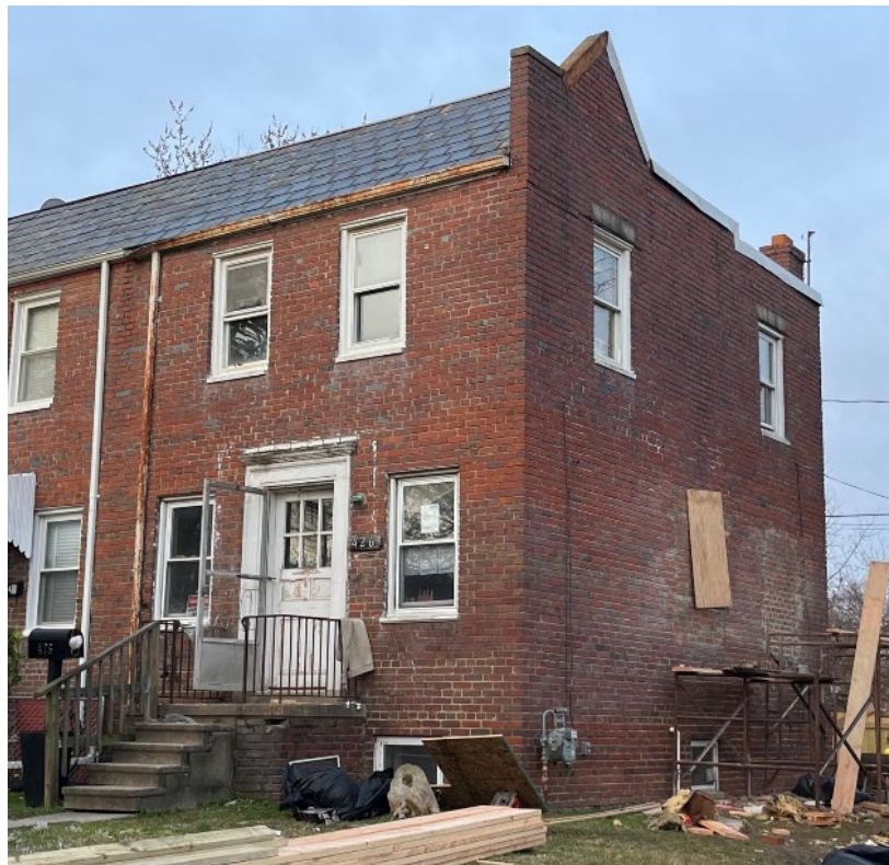
Figure 1: Modifications made to the north elevation without BAR approval
