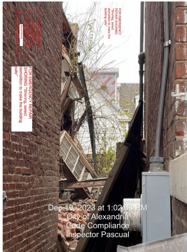
Figure 1: Ell east elevation post collapse; main block in foreground on left.
