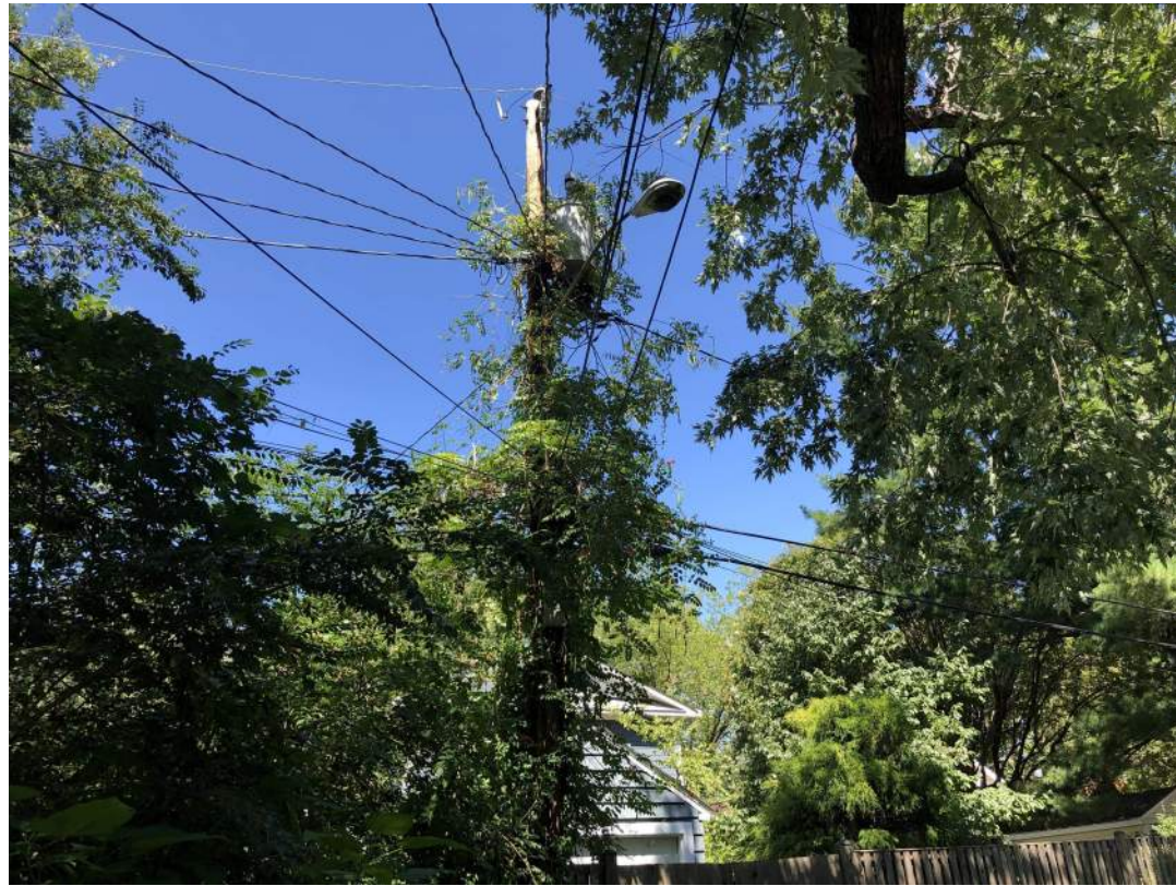
1. EXISTING UTILITY POLE FOR HOMES AT 1405 TO 1411 MT. VERNON AVE. & 404 TO 406 E. ALEXANDRIA AVE.
