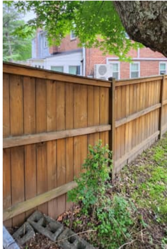
Elevated HVAC unit.
