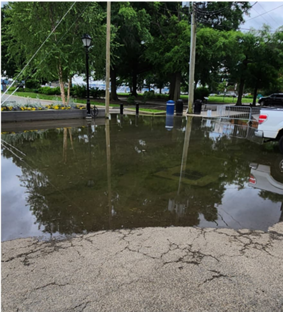
Ponded water at storm drain inlet.
