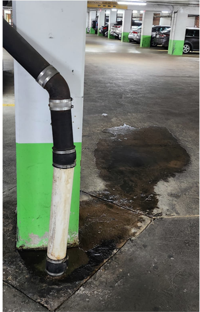
Leakage of roof drain.
