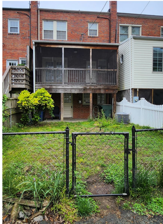
Basement entrance and HVAC unit susceptible to flooding.
