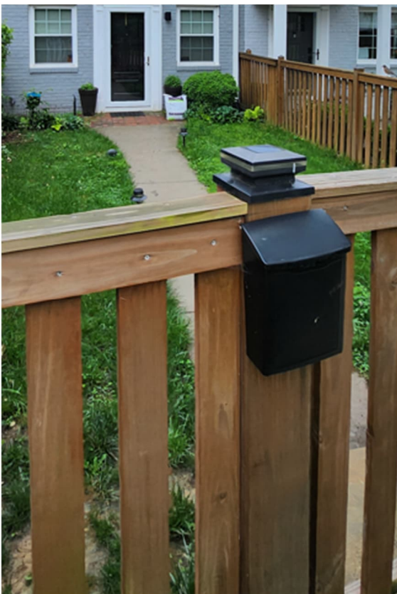
Front of structure susceptible to flooding since sidewalk is higher than structure's walkway.
