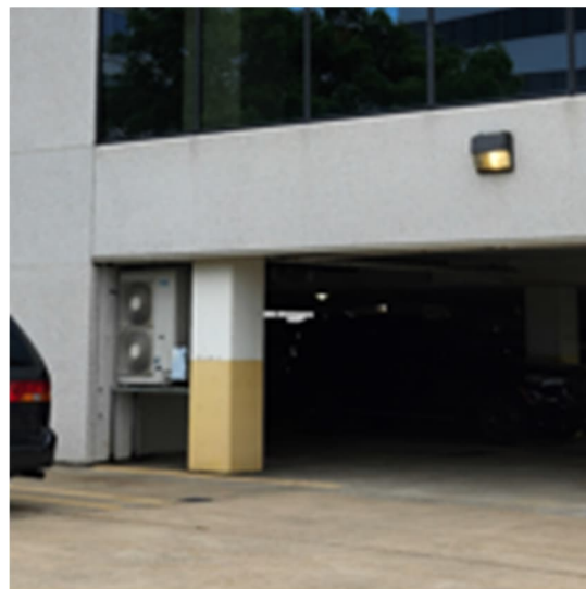
Elevated utility unit.
