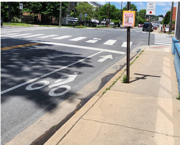
Standing water along curb & gutter.
