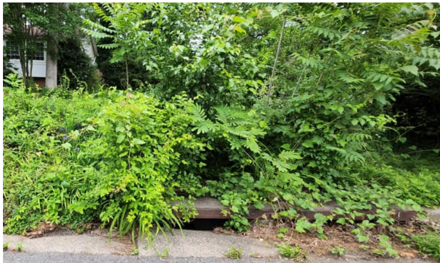
Storm drain inlet blocked with leaves and debris.
