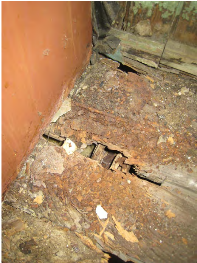
Figure 8 – Condition of floor and framing in existing rear “el” addition
