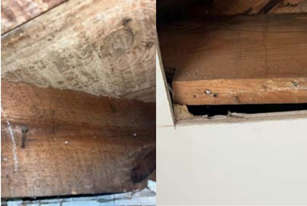
JOIST PHOTO FROM THE ADDITION (EASTERN WING OF THE SINGLE FAMILY HOME TAKEN FROM THE BASEMENT/LOWER LEVEL)
