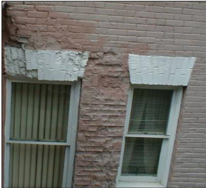
Photo of spalled/damaged brick due to moisture
