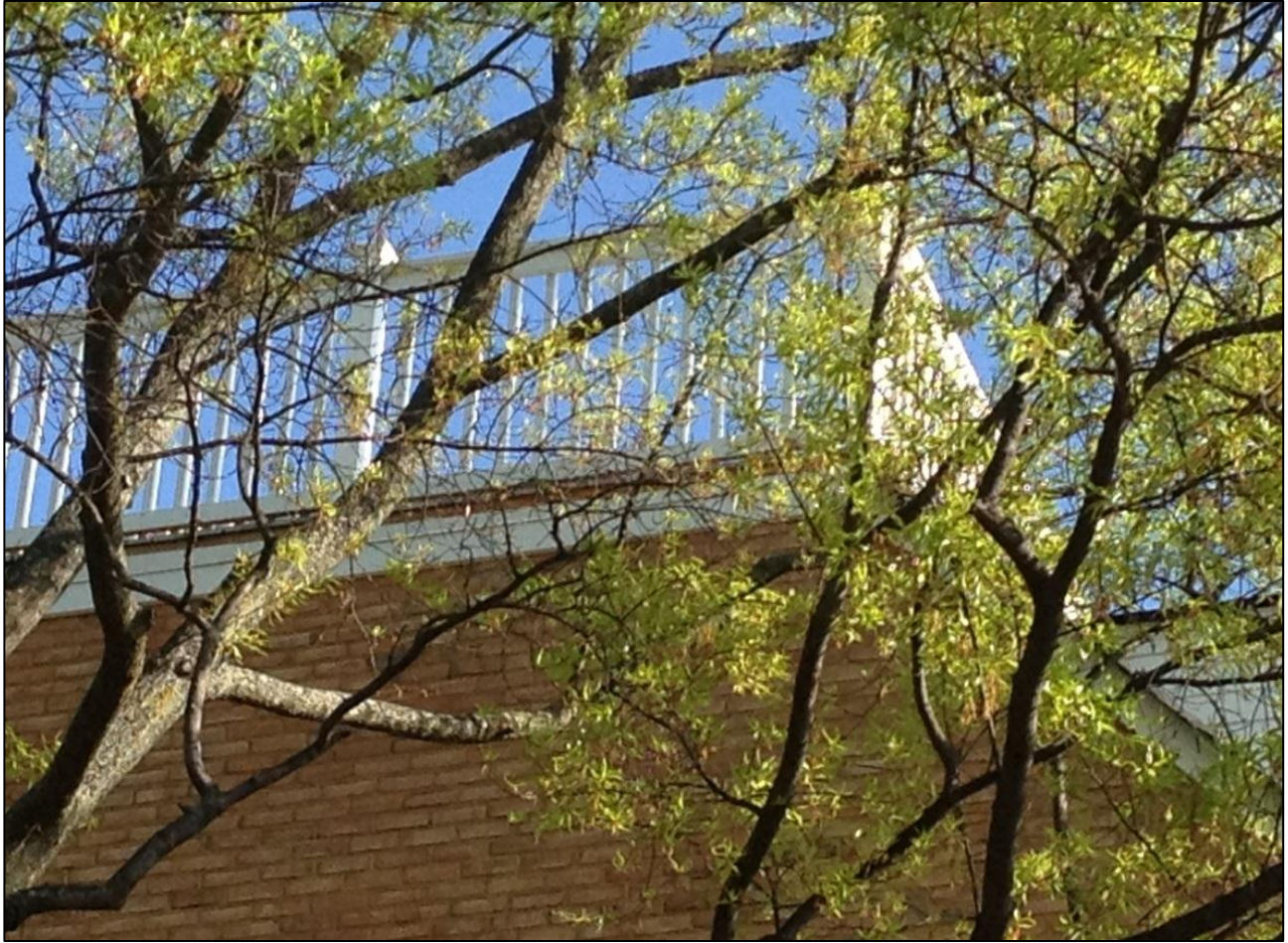
Roof deck railing, as constructed, with narrow posts instead of the wide plinths
