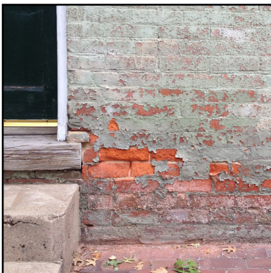
Rising damp (water wicking from below) has caused the face of this early brick to crumble from the freeze-thaw cycle.
