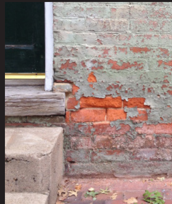
Rising damp (water wicking from below) has caused the face of this early brick to crumble from the freeze-thaw cycle.
