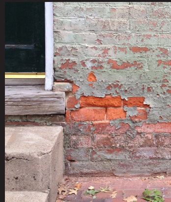
Rising damp (water wicking from below) has caused the face of this early brick to crumble from the freeze-thaw cycle.
