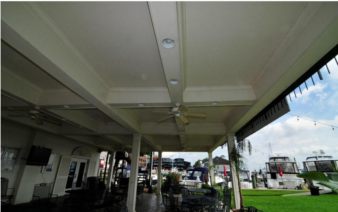
Figure 41: East Façade, Looking North on Patio Added in 1967, Renovated in 2002 (Thunderbird Archeology 2016)
